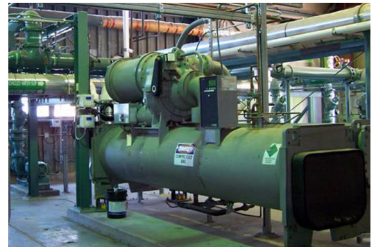
Chiller equipment used at the Performing Arts Center. Photo: Cal Poly Engineering Services.
