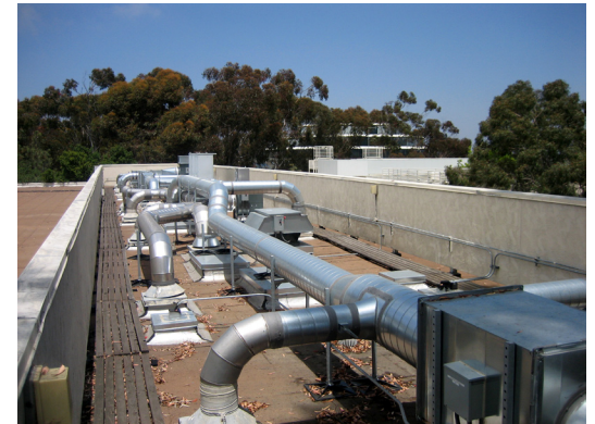
View of the interconnected ductwork and new exhaust fans. Photo: John Dillriott.
