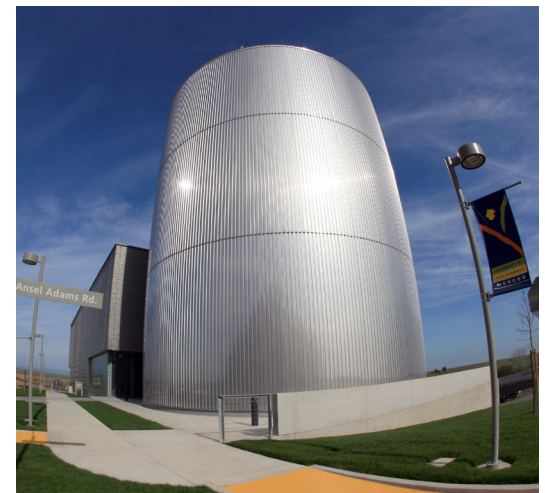
View of the campus's two-million gallon thermal energy storage tank. Photo: UC Merced.
