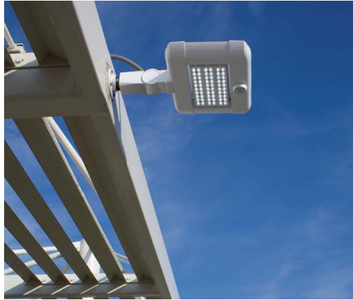
LED lamp attached to parking structure. Photo: CLTC
