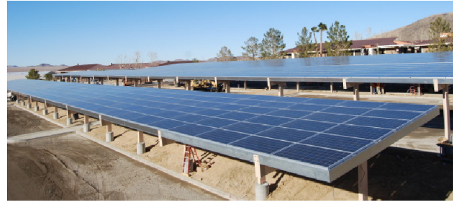
View of photovoltaic array integrated into parking shade structures under construction in 2010. Photo: CMCC.
