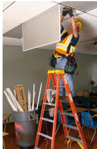
Copper Mountain College replaced all interior and exterior lighting fixtures. Photo: CMCC.
