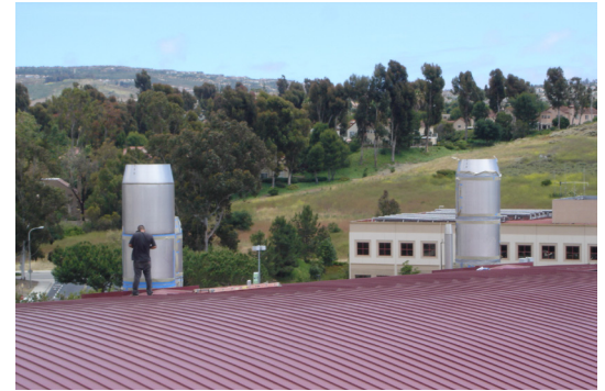
Exhaust stack extensions installed at Croul Hall. Photo: UC Irvine.
