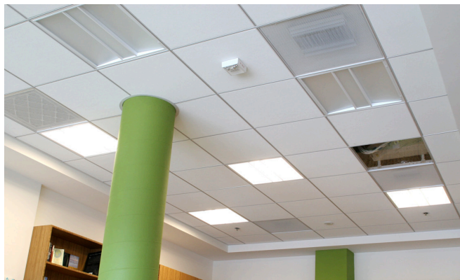
View of the lighting system, with electrified grid, and clear view panel. Photo: UC Regents/Rhett S. Miller.
