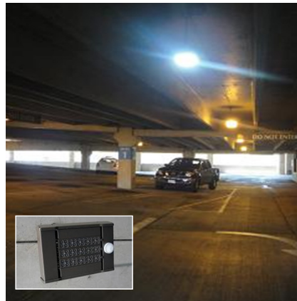
New LED fixtures installed in Parking Structure 1. Images: CSU Long Beach.
