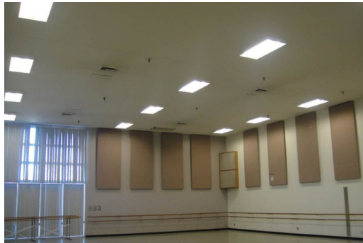
High-bay T5 high output lighting in the School of Dance. Image: CSU Long Beach.
