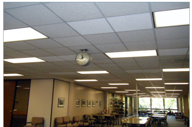
The lighter ceiling tiles show where fixtures were removed during the retrofit. Image: CSU Chico.
