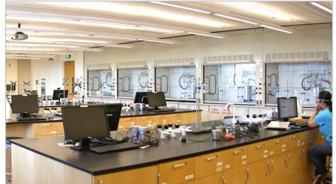
The Naraghi Hall retrofit reduced ventilation rates during times of low and no occupancy. Image: CSUS.
