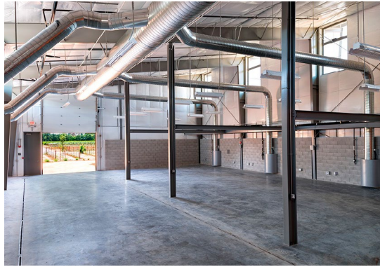
View of interior shows displacement diffusers inside the partial height CMU wall. Photo: Jasper Sanidad.
