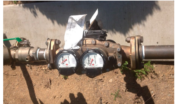
Compound water meters were installed to accurately measure low and normal flow rates. Photo: Ed Johnson.
