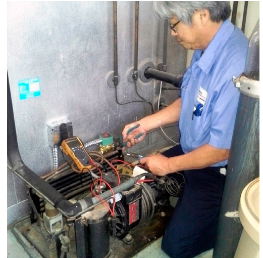
Performing an in-house custom retrofit for a cold-room condensing unit. Image: Danny Paik.
