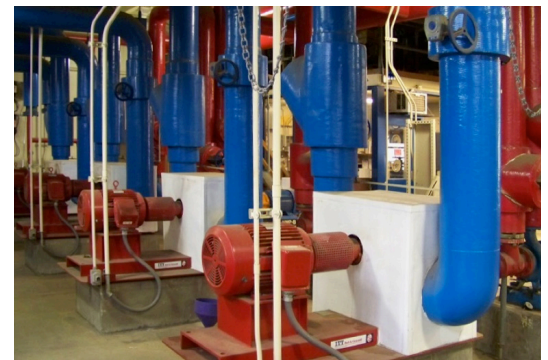
Central pumps for hot and chilled water present opportunities for significant energy savings. Image: Geng Liu, CSU Stanislaus.
